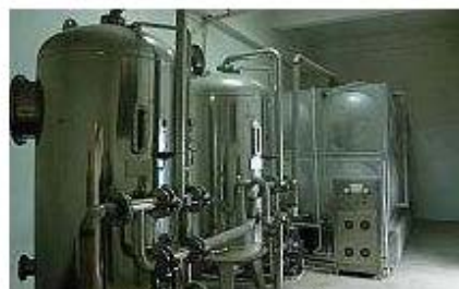
Water re-use facility
