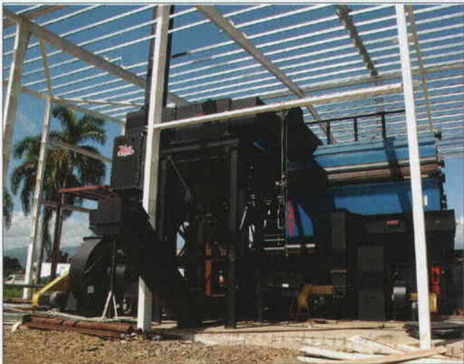
This biomass plant in the Dominican Republic is under construction on the site of HanesBrands' textile fabric plant in Bonao.
